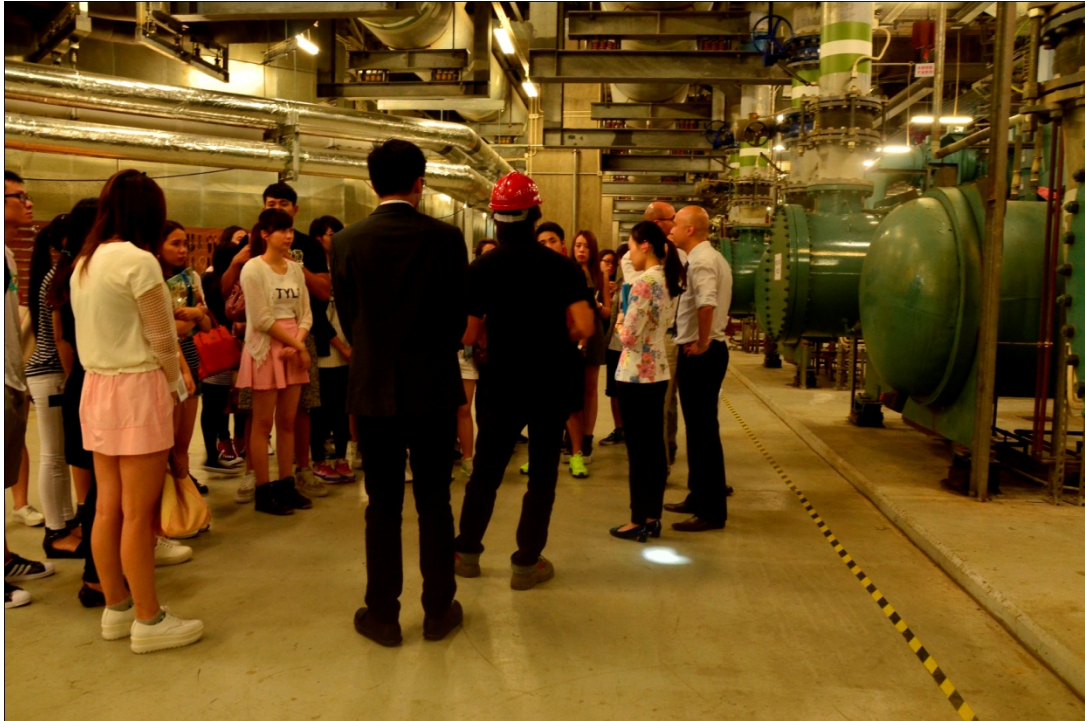
P004: Students paid a visit to the central chiller plant which helps reduce the energy consumption of the air-conditioner unit.
